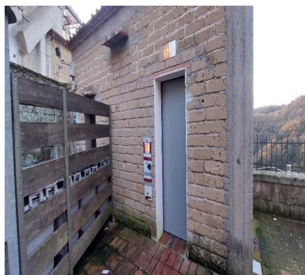
77 public toilet door with coin mechanism and contactless card device
