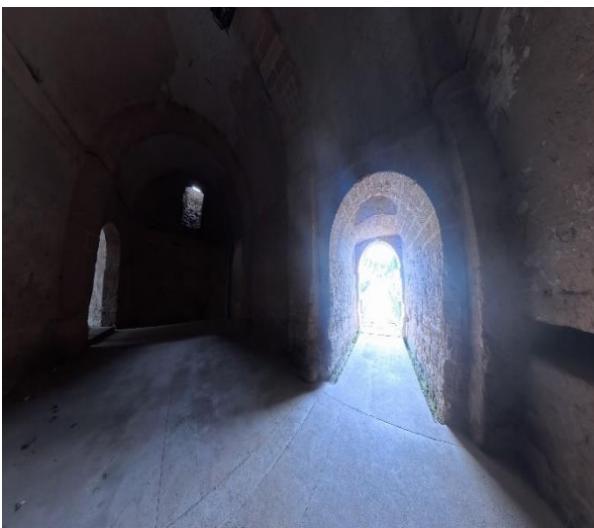
58 First Access Door
